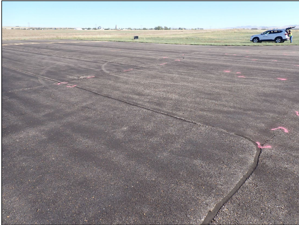
TW-03-04: L&T Cracking
