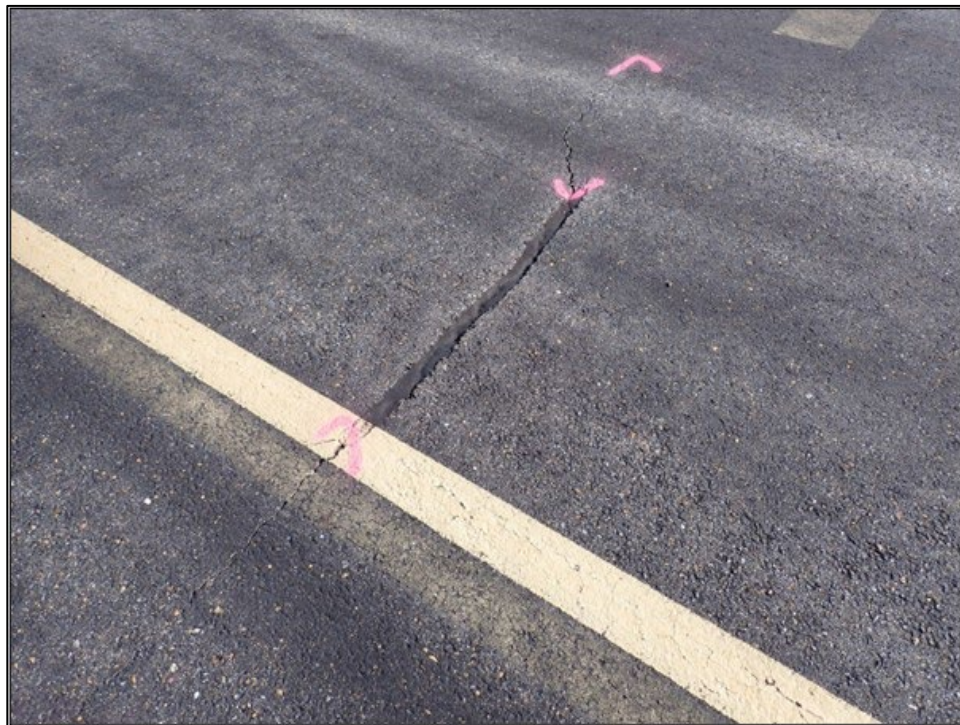
AP-02-02: L&T Cracking
